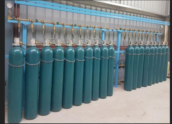
Gas Manifold System
