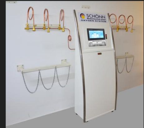
Medical Gas Manifold System
