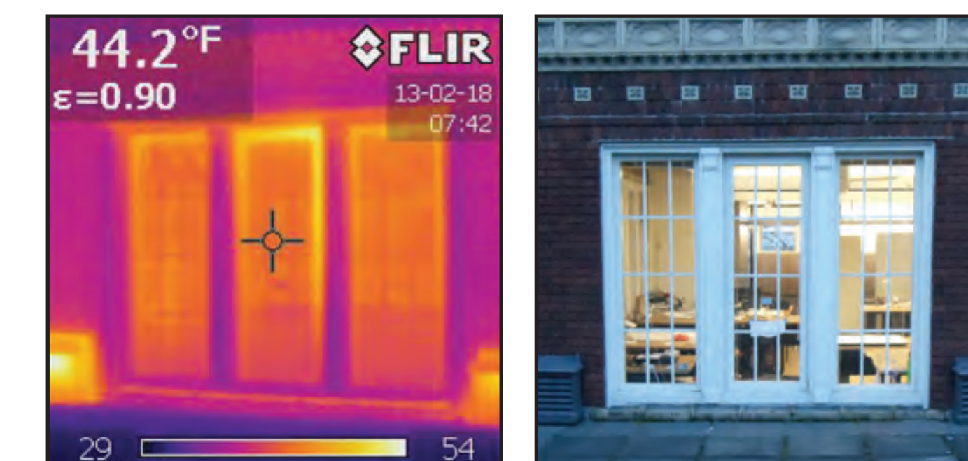
Figure 2.2 - Shattuck Hall post-retrofit 1986. has a leaky frame thermally bridging a rate that keeps the exterior facade an average 7.4°F higher than the ambient outdoor air.
