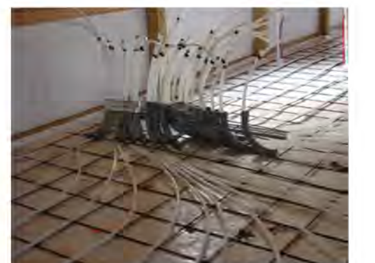
Radiant Heating and Cooling
