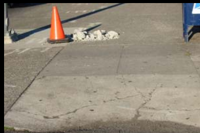
D. Cracked Concrete
