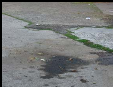
B. Damaged and Oil
