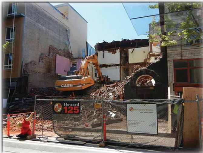
An old building being torn down. It used to house the legendary Satyricon nightclub.
