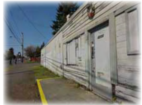
I don't like the fact that these building is abandoned and not used for nothing. It could benefit us by being a gym with a pool where it could help us physically by moving in where we could get exercise. Also we could hang out with our friends and at the same time we could relax and get healthier (Blanca).
