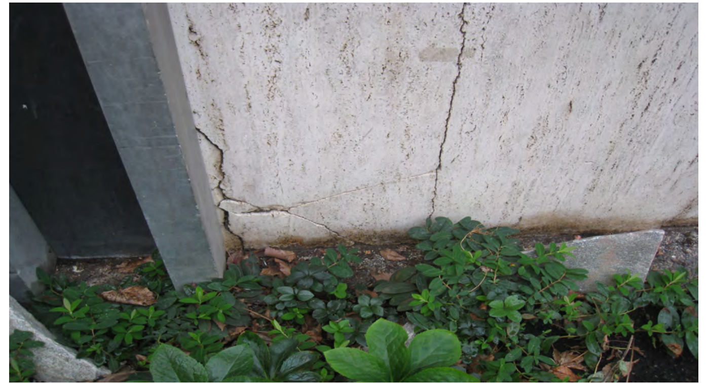
Figure 16 Broken Travertine Wall Panels
