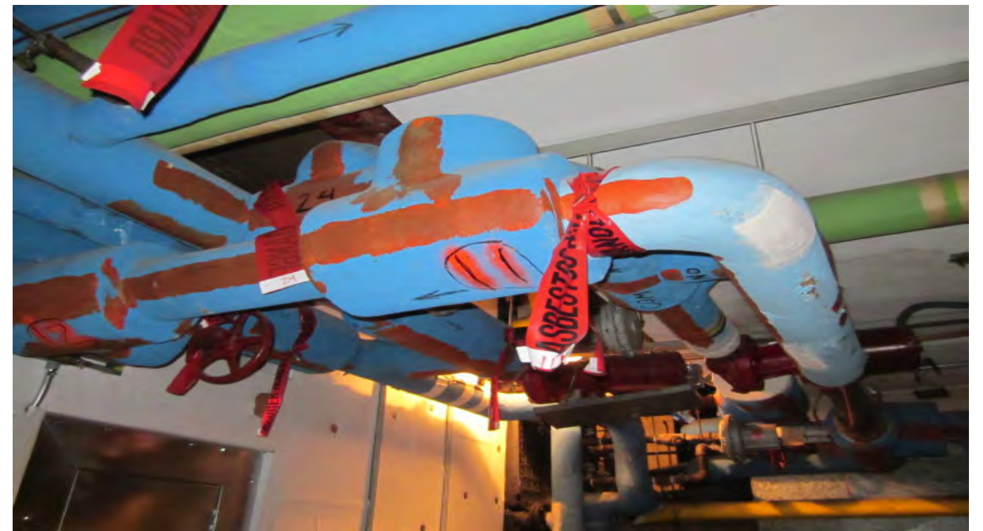
Figure 13 Asbestos Pipe Insulation Throughout
