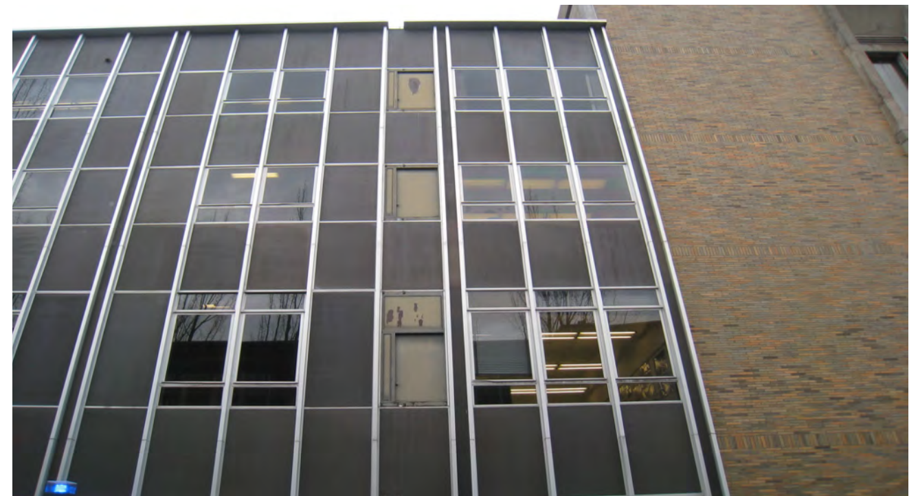
Figure 15 South Maintenance Doors Without Fall Protection
