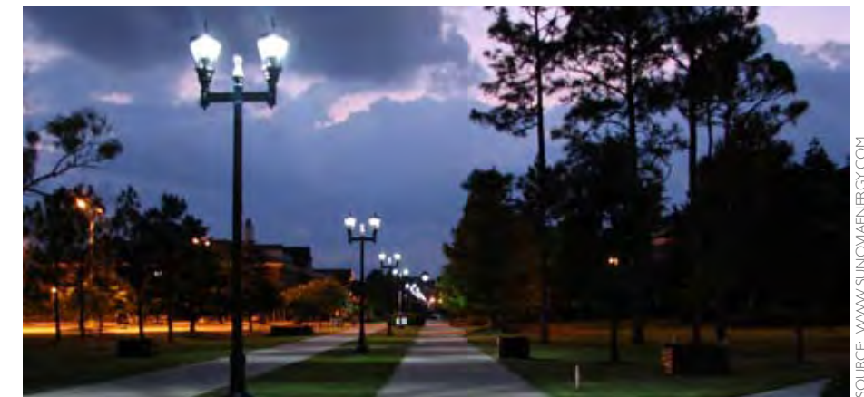
LED lighting along a streetscape.
