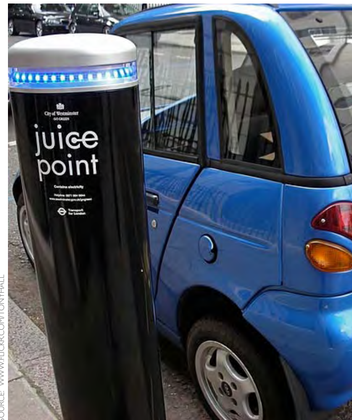
“Juice Point” or electric car charging station.
