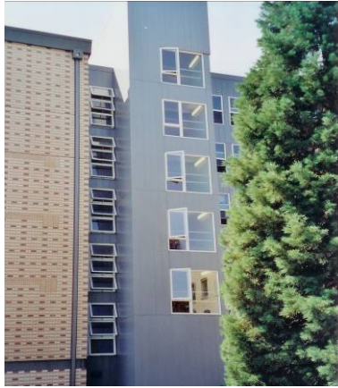
Figure ES-2: East side ventilation. (7/2004)
