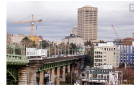
Cranes tower above Seattle's University District neighborhood as a building boom continues there. (Elaine Thompson / The Associated Press)
