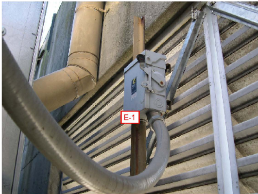
Cooling tower disconnect
